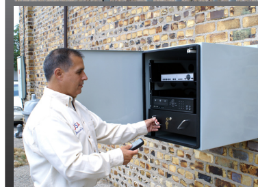
Rack Enclosure mounted on a wall
