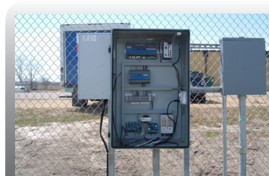
Along a gate using metal tubing to run wiring from one enclosure to another
