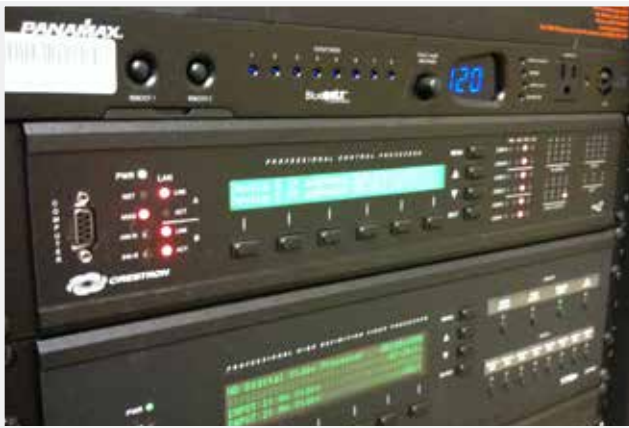
Panamax BlueBOLT-enabled M4315-PRO's are integrated with Crestron Control Systems at SLU to facilitate local and remote power control and monitoring.
